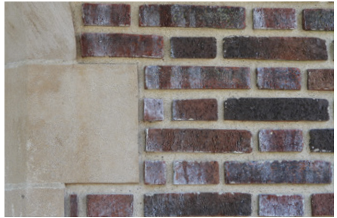
▲ As part of the overall exterior repairs, all the mortar joints between the bricks and limestone were replaced.
